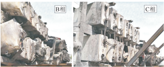
图10 B相、C相并联电容器组损毁情况 Fig. 10 Damage situation of phase-B and phase-C capacitor bank
